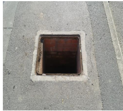
Missing Chamber Cover
