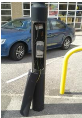
Lighting Column access cover Removed exposing cables
