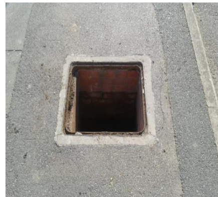
Missing Chamber Cover
